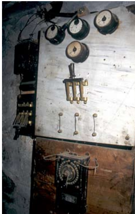
Panel de control.
